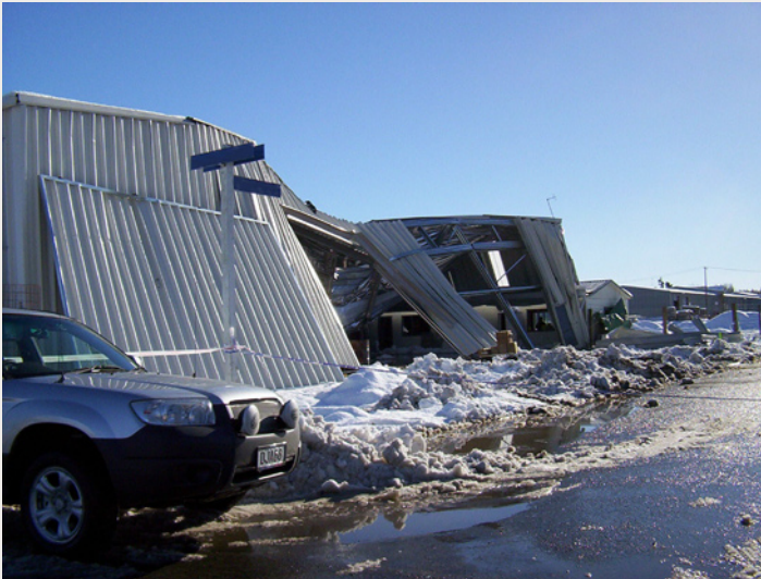
“The weight of snow was too much for this building in South Canterbury”
