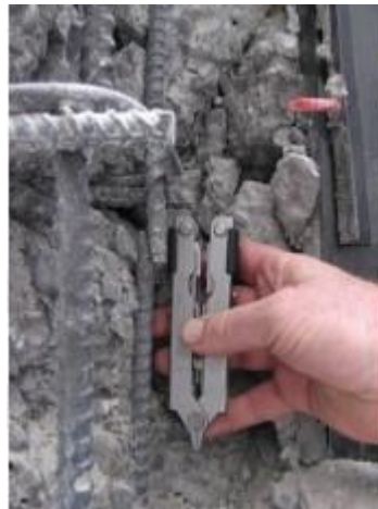
Figure 6: Fractured bars in lightly reinforced wall
