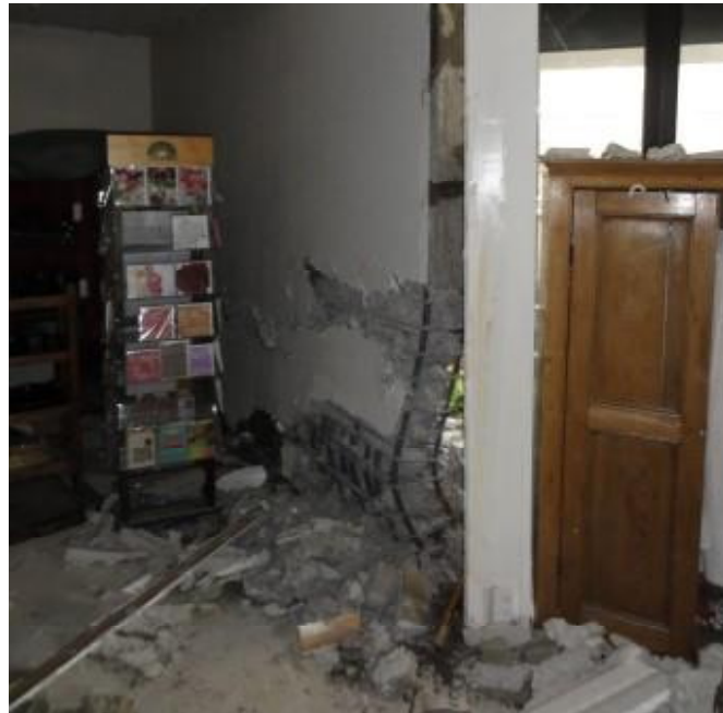
Figure 4 Buckling of concrete wall with confined boundary regions
