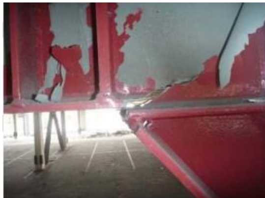
Figure 10: Fabrication eccentricity causing fracture of EBF
