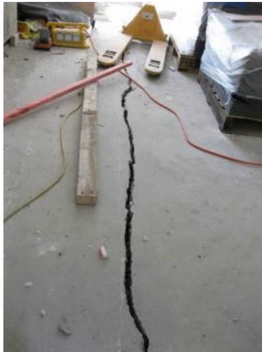
Figure 9: Floor tearing caused by frame elongation
