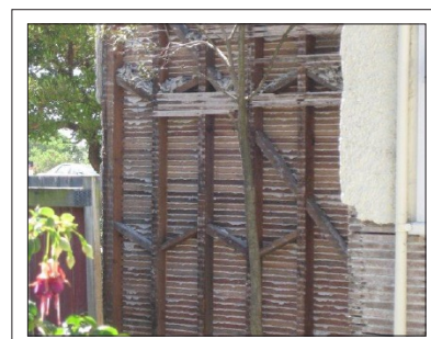
Figure 3: A failure example of lath and plaster wall [5].
