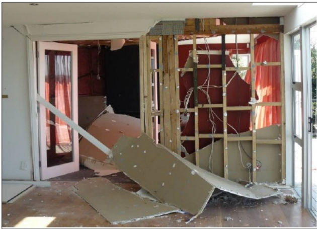
Figure 37: A severe failure of the plasterboard internal linings after the 2011 Christchurch earthquake [5].
